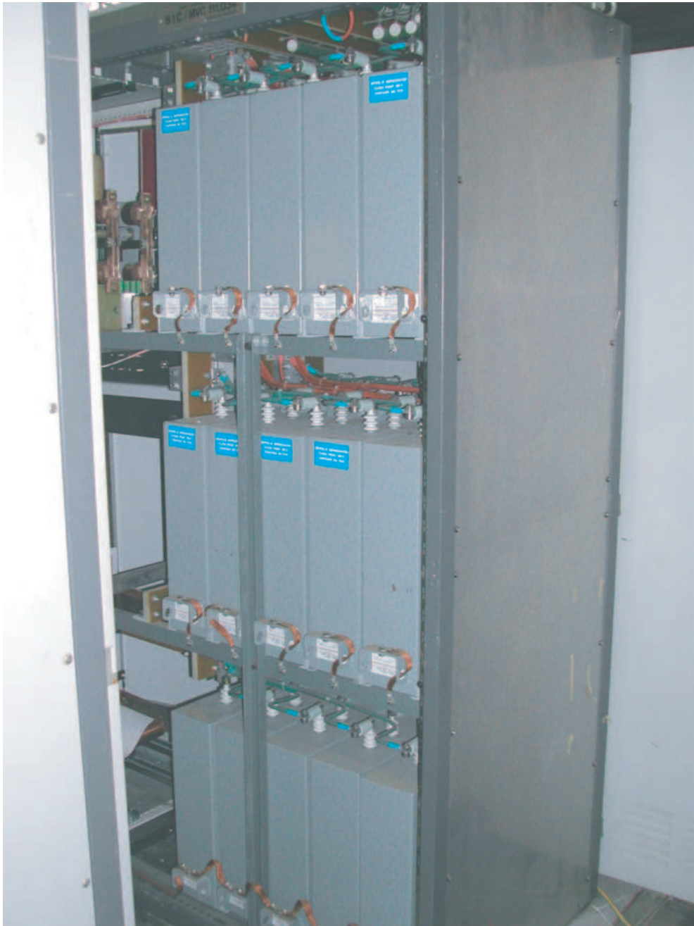
Figure 3.17: Set of capacitor banks used for the discharging circuit. The discharging circuit is located in front of this unit.
