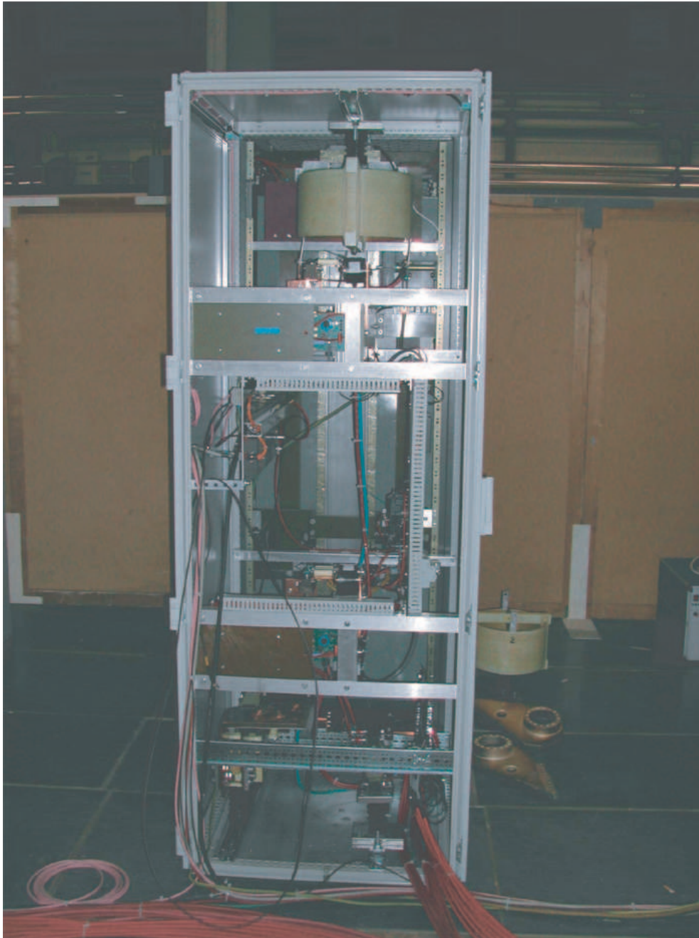
Figure 3.16: One of the two units of the discharging circuit. At the right bottom corner the red cables are connected to the horn. The capacitor banks are located behind this unit.
