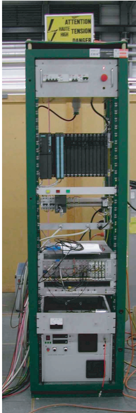
Figure 3.19: Power supply controller rack. From the bottom to the top: high voltage charging unit, timing circuit, controller, electric switches.
