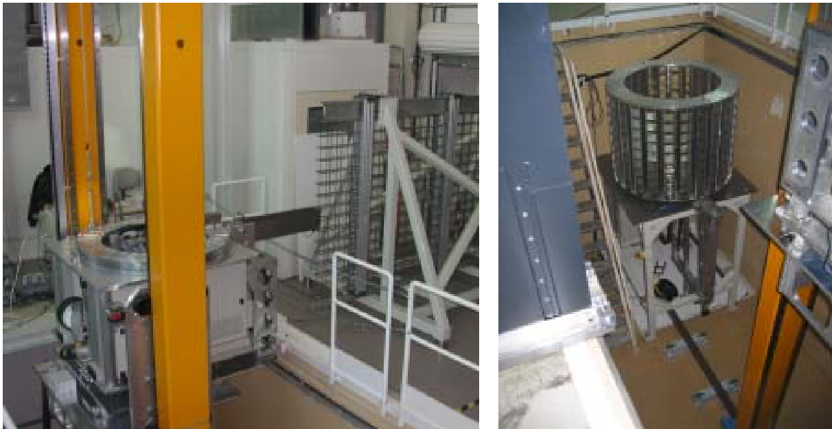
Figure BMS.3: pictures of the first manipulator being tested in Annecy. On the left, the portico (yellow pillars) with the platform is docking a brick supporting wall section prototype. On the right, the loading station of the system can be seen with its revolving basket on top.
